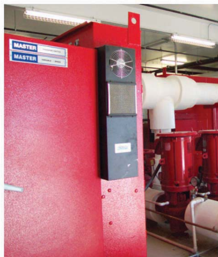
photo courtesy of Master Controls
