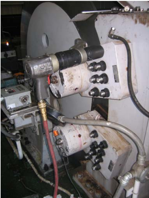
BRAKES ON A GANTRY SHIPPING CRANE WINCH AT SHIPPING PORT
