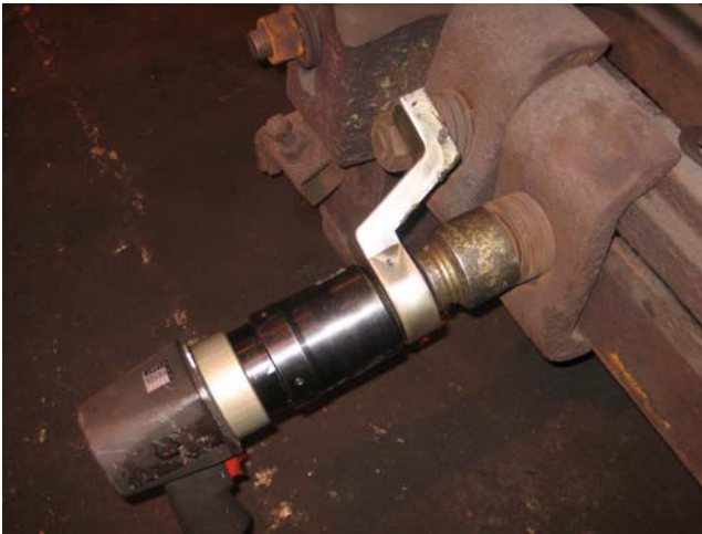
ROLLING MILL GUIDE RAIL BOLTS
