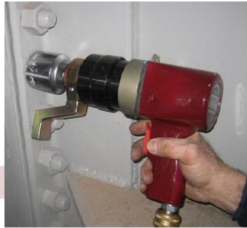
AT1000R ON A STEAM CONDENSOR (Power Gen)
