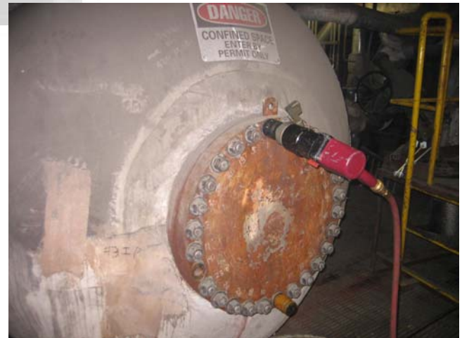
HIGH PRESSURE VESSEL IN A POWER PLANT
