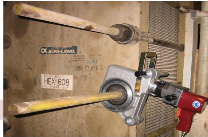
PLATE HEAT EXCHANGER BOLTS
